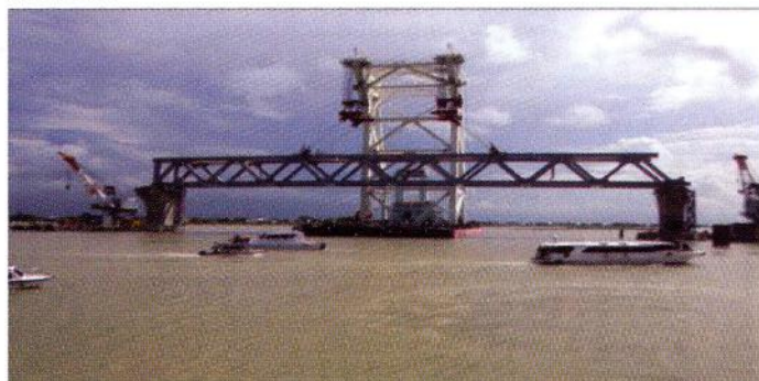
The much awaited Padma Bridge becomes visible as the first span installed between pillars 37 and 38, 30 September 2017.
